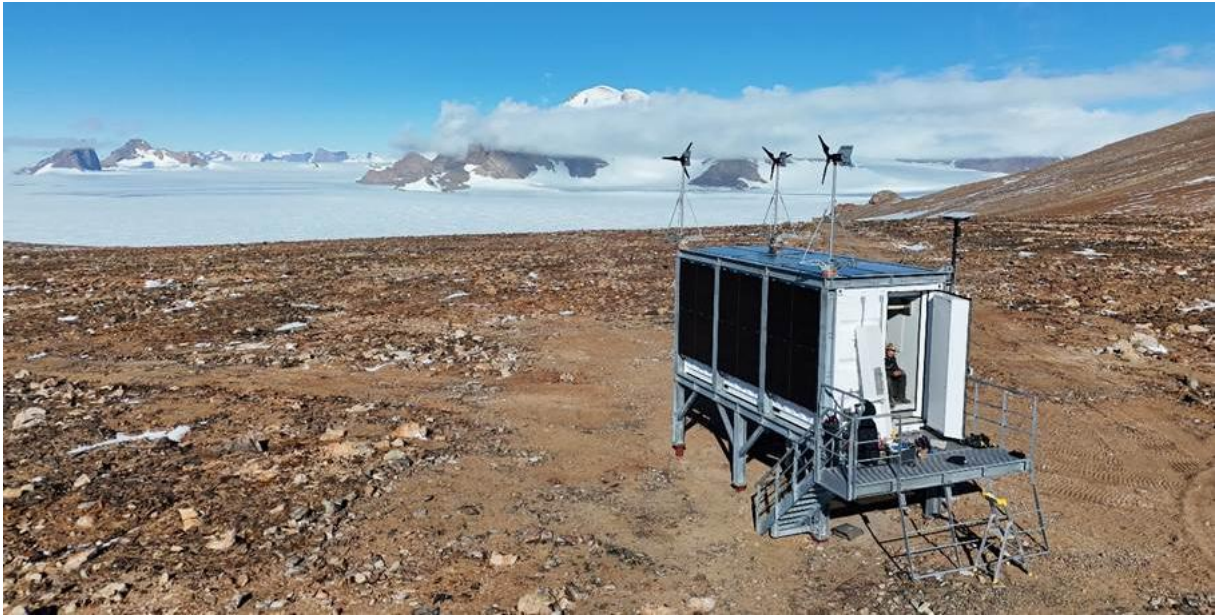
The Central Recording Facility (CFR) installed with windmills, solar panels, and communication antennas at Armlenet. Photo: NORSAR.
